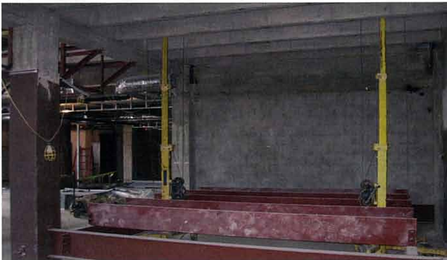
Construction filters were placed on all HVAC ductwork so the building's occupants wouldn't be exposed to dust from the construction. Photo: Bailey Architects.
